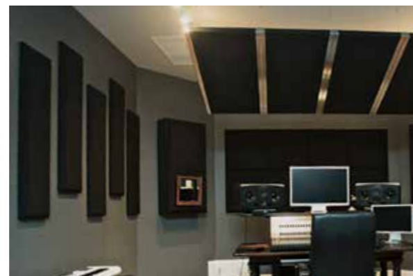
Primacoustic studio installation
